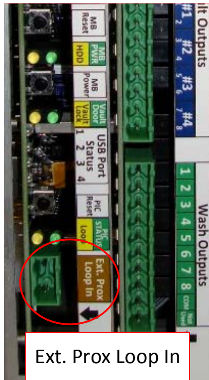
Figure 28. External Prox Loop Lead-In Connections
