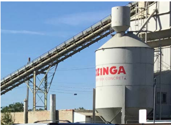
Existing Industrial Equipment at Ozinga Cement Plant in Wheeling.
