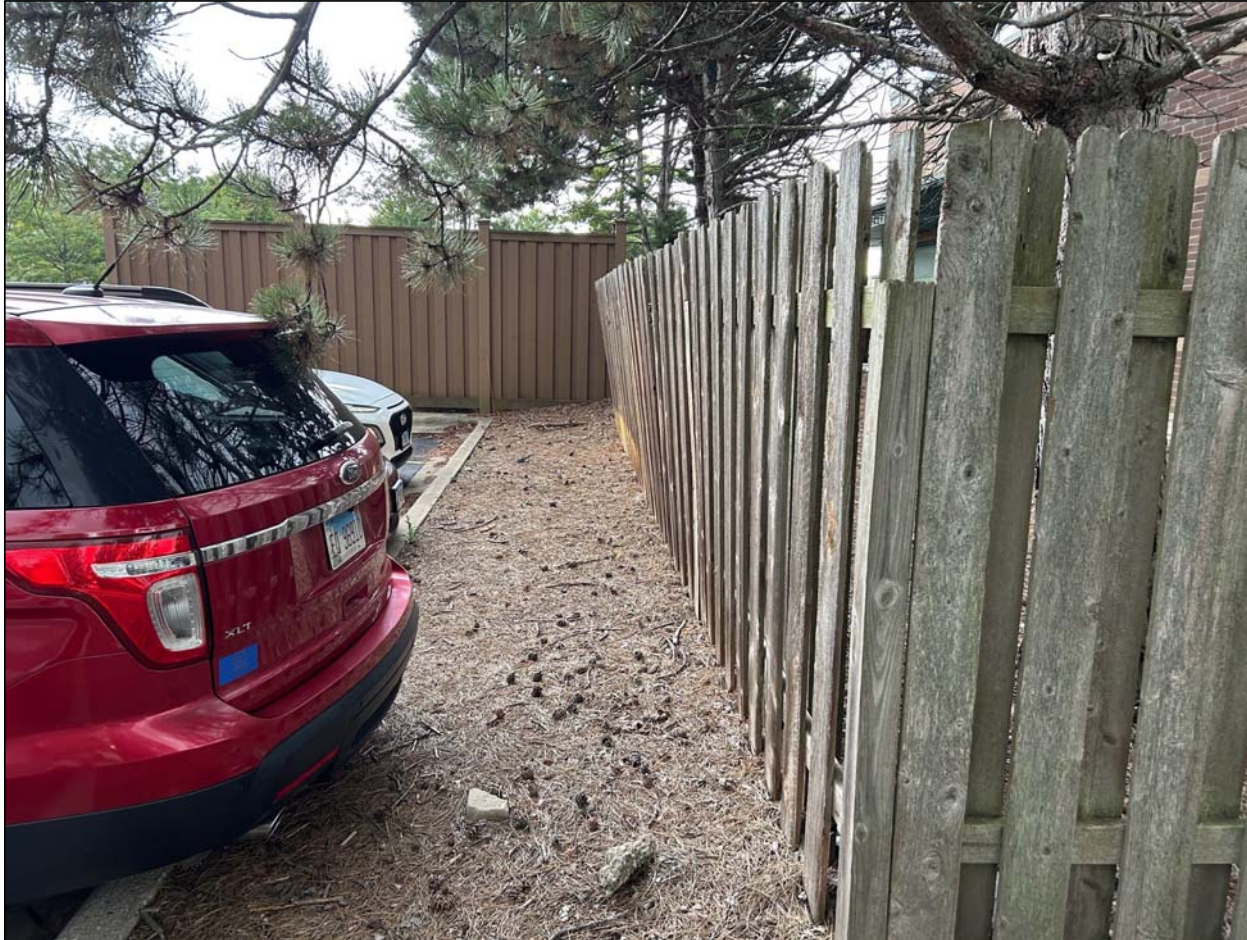
Photo of the fence along the east property line that needs repair.
