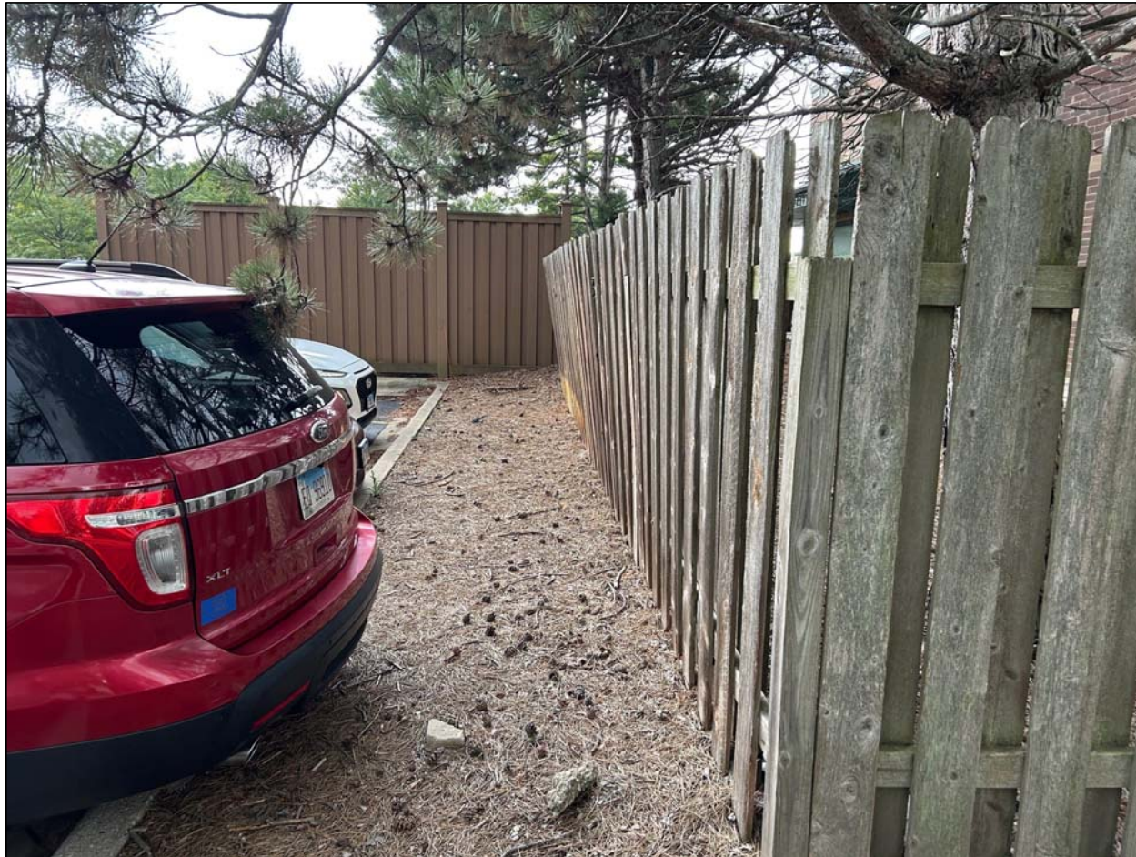
Photo of the fence along the east property line that needs repair.
