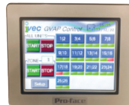
HMI Central Control Home Screen
