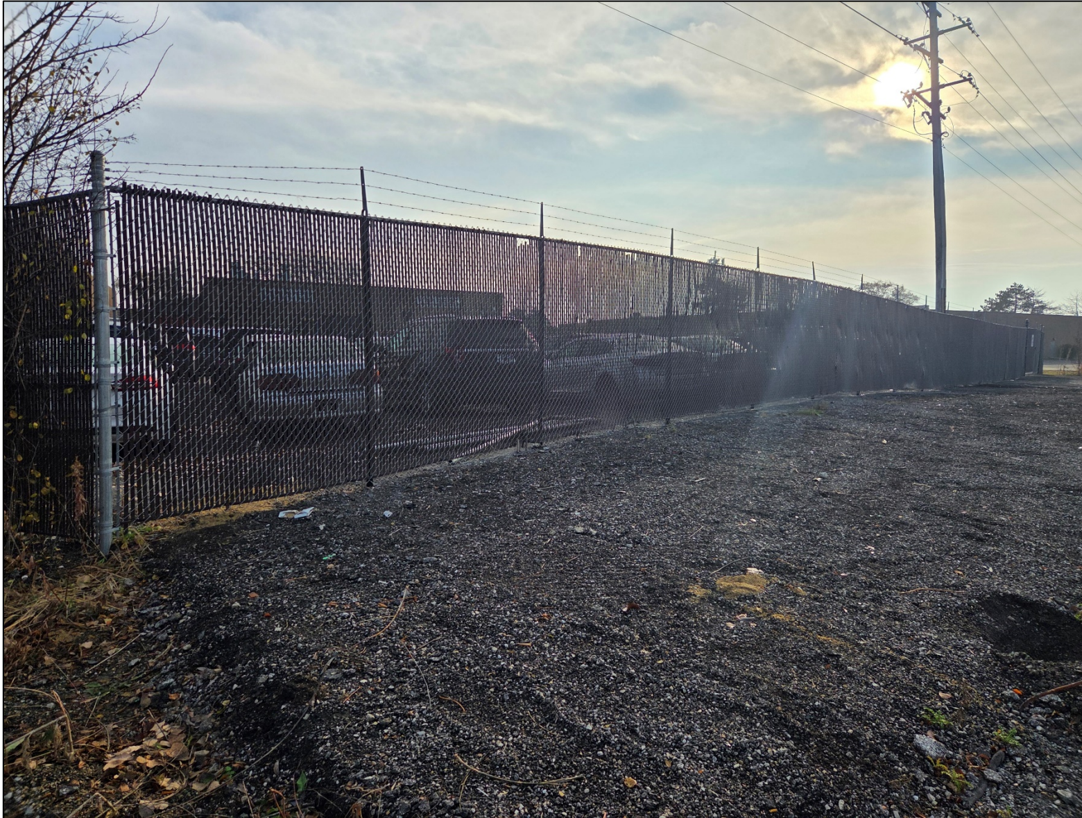
Photo of the new fence on the west property line taken from ComEd property.
