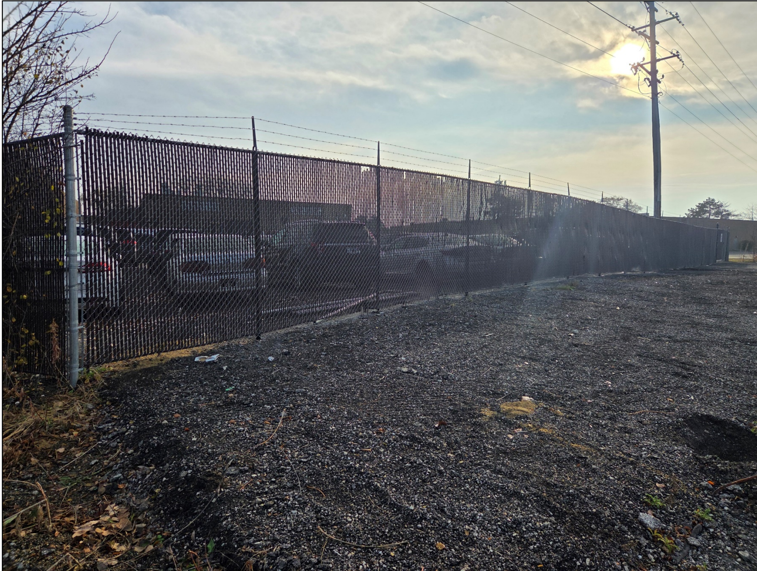
Photo of the new fence on the west property line taken from ComEd property.
