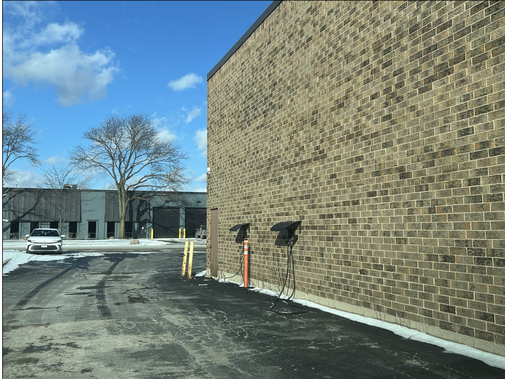
Existing Non-Permitted EV Chargers Mounted on West Building Façade – To Be Removed.
